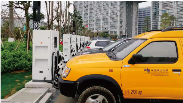
Guangdong Power Grid PV-ESS-EV Charging
