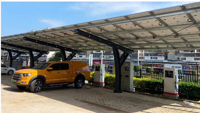
State Grid PV-ESS charging discharging inspection station V2G
