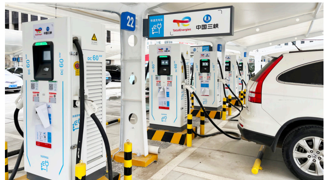
Changxia Expressway (TotalEnergies & Three Gorges Corporation) Public Charging Station Mobility Hub
