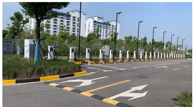
Shanghai Tobacco Group Charging Station Workplace Charging
