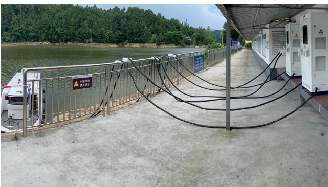
China State Shipbuilding Corporation Onshore Charging
