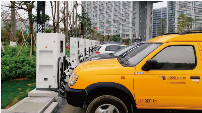
Guangdong Power Grid PV-ESS-EV Charging
