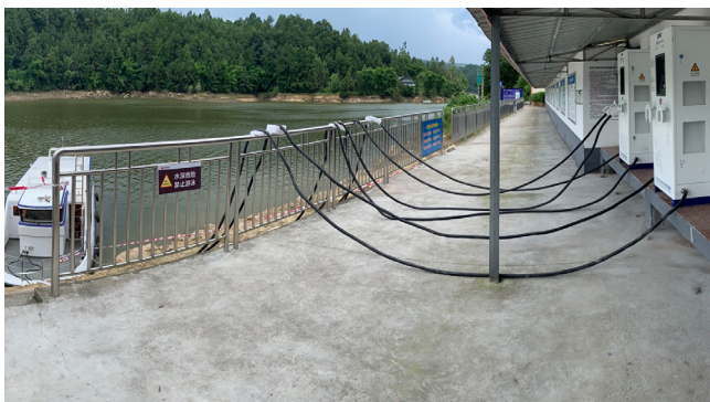
China State Shipbuilding Corporation Onshore Charging
