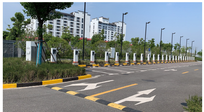
Shanghai Tobacco Group Charging Station Workplace Charging
